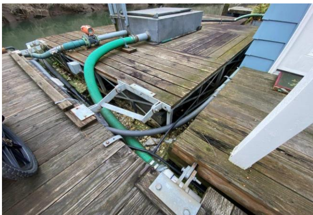
Sewage Ejection/Lift System-Pumps- Replace
