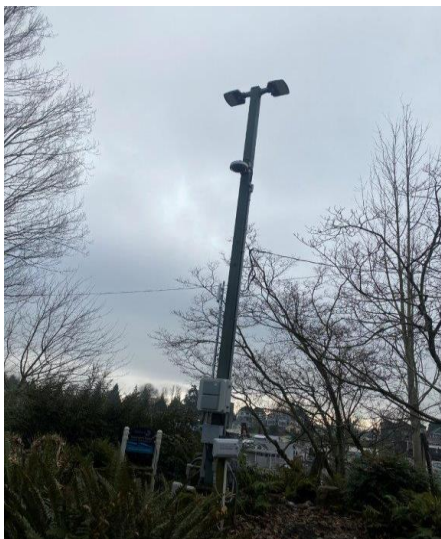
Lights-Exterior-Pole-Parking (Heads Only)
